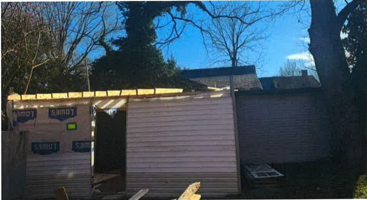
This is how the building looks from the front. And how uniform the exterior walls will look with the existing wall. They will be painted to match the house.
