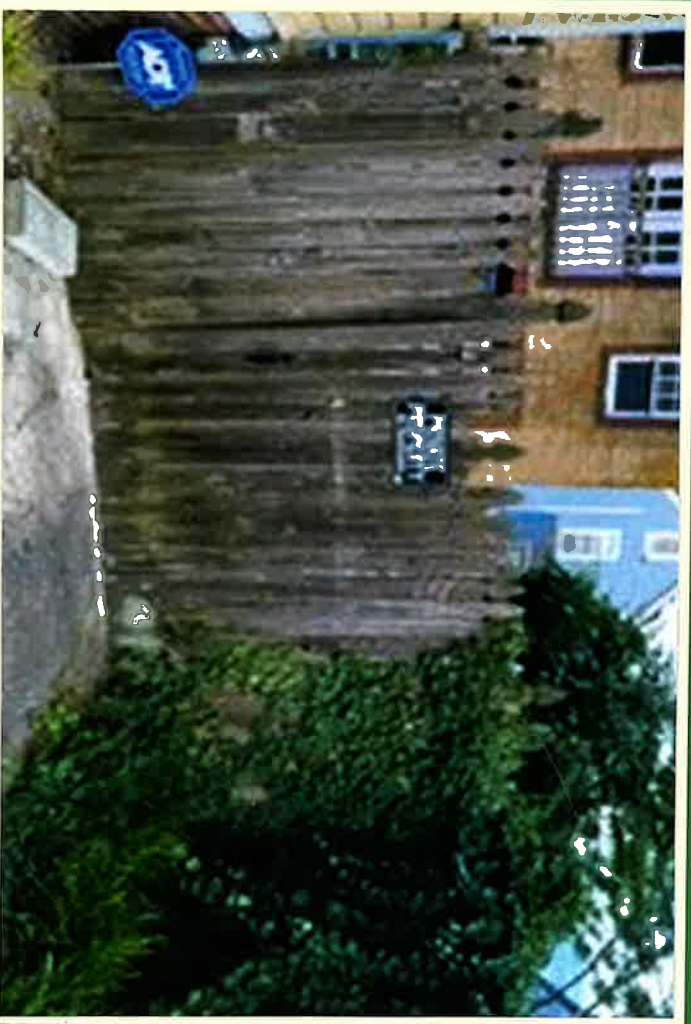
Front gate to be replaced
