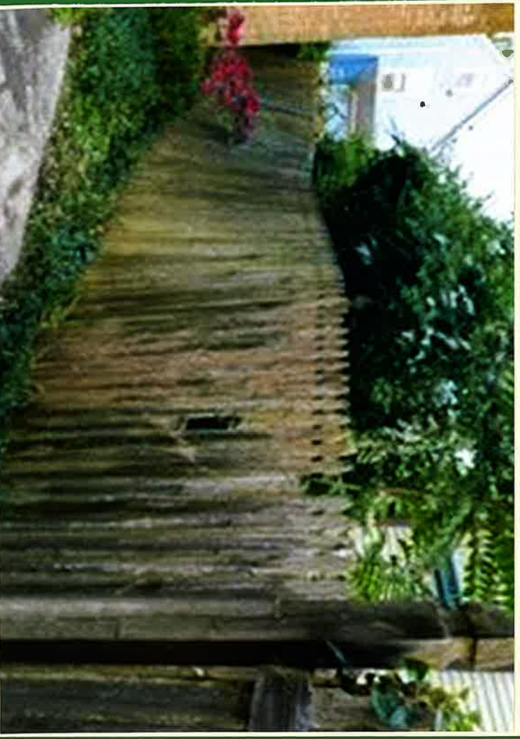
Right side fence to be replaced
