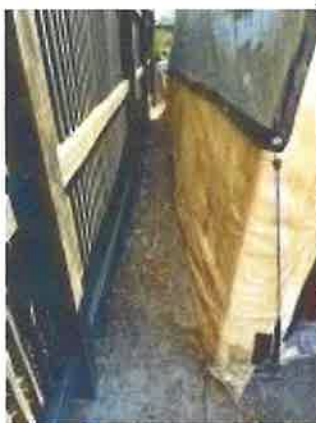
Old Garage Left side Slab
