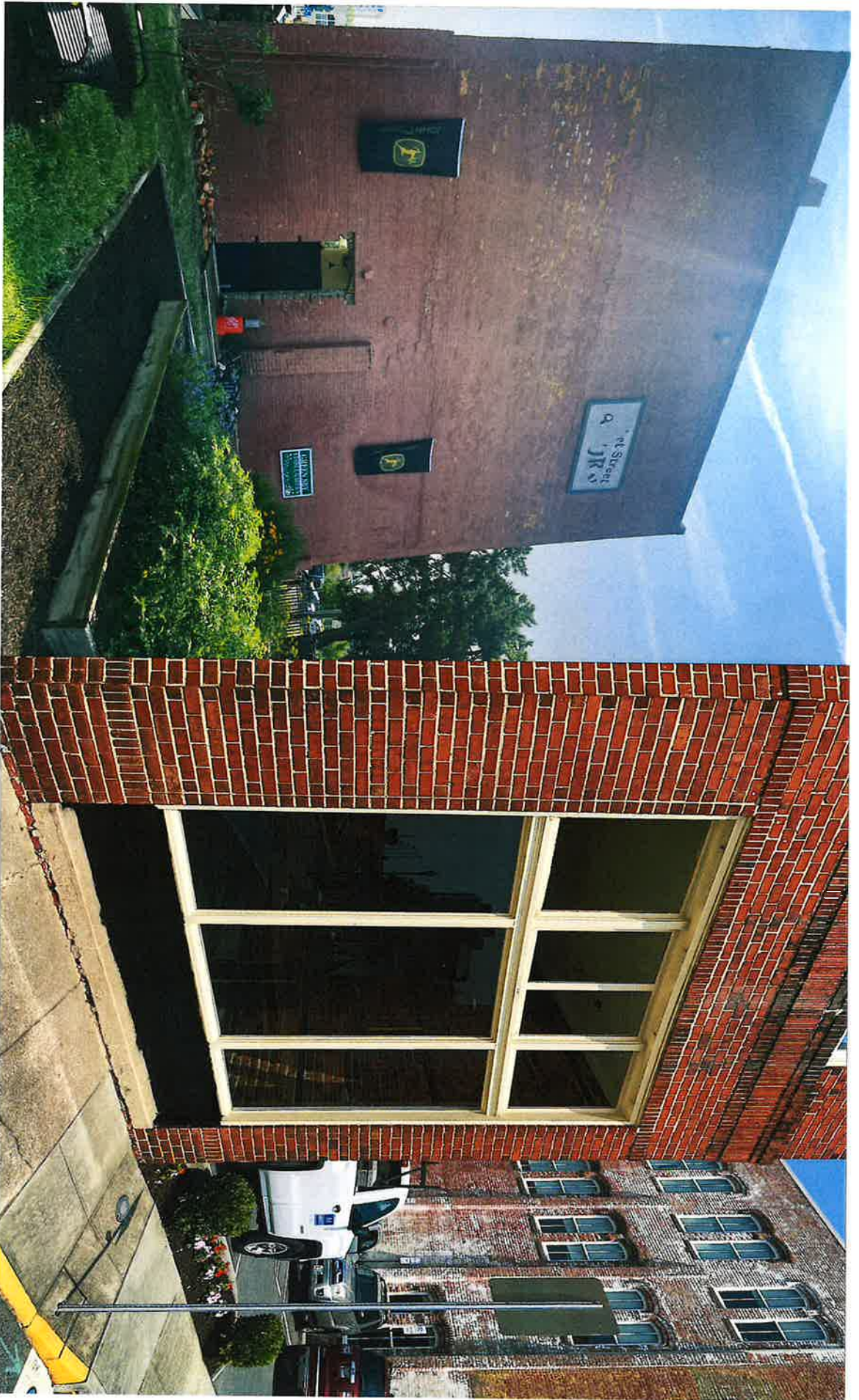
View from Salisbury eatable gardens showing damaged door
