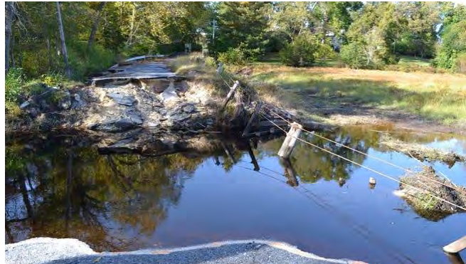
Photo 2. The dam and road at Barren Creek Pond failed during a severe July 2016 storm. The County rebuilt the roadway but did not restore the dam. Photo by Liz Holland.
