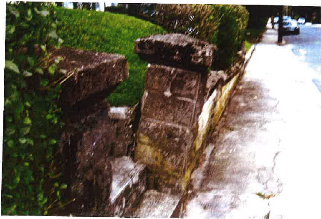
SHOWING LEAN OF THE WEST SECTION OF THE RETAINING WALL
