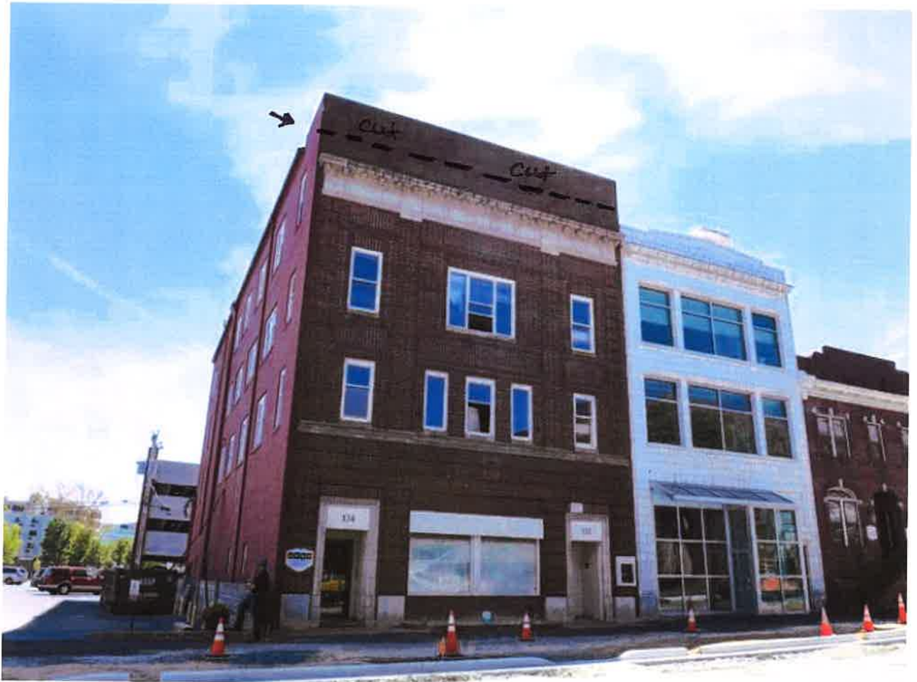
132-134 E. Main St Proposed removal of bricks
